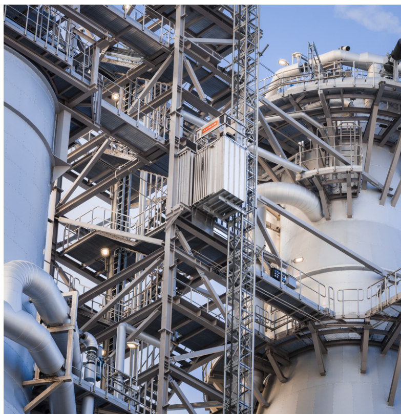
The Alimak rack-and-pinion elevator is used approximately 25 times per day for service and inspection of the pulp mills boiler.
