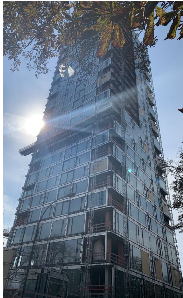
One out of eight Alimak MC 450 mast climbing work platforms at work on the 160 Park View construction project in Frankfurt am Main, Germany
