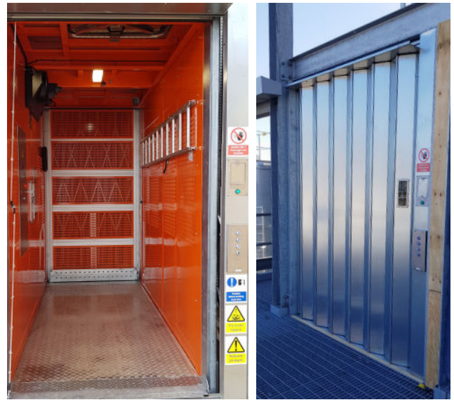
Data Center, Slough, United Kingdom
